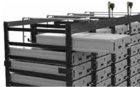
Images C - Suppression system injecting Forrex cooling agent into battery modules
