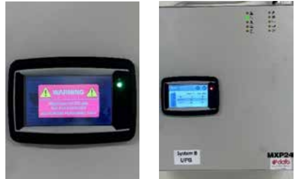
Images H – system power supply (UPS) with touchscreens for service and OPC UA gateway
